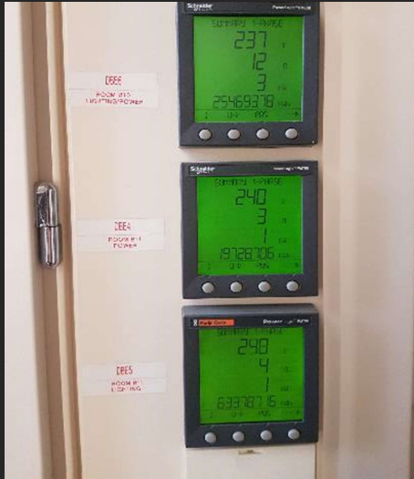
Electrical power readings
