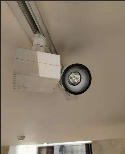
Existing Halogen lighting
