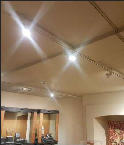
Existing lighting, no occupancy controls
