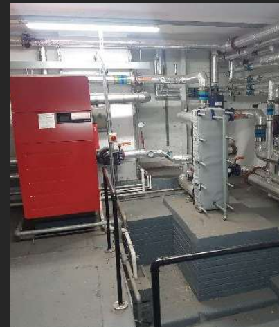
Gas boilers, opportunity to reduce heating water temperature
