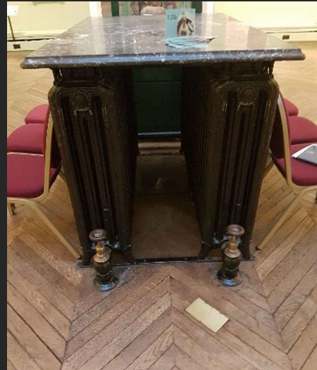
Existing radiators do not have thermostatic valves
