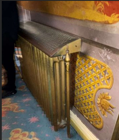
No valves on existing radiators
