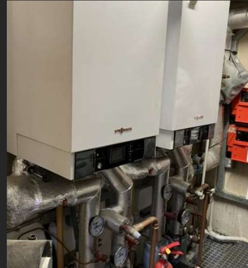
Gas boiler, consider replacement with heat pumps
