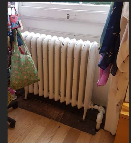
No valves on existing radiators
