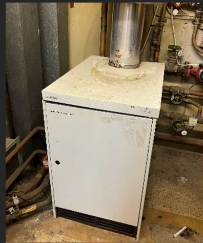
Existing gas boiler
