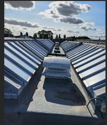
Opportunity for PV panels
